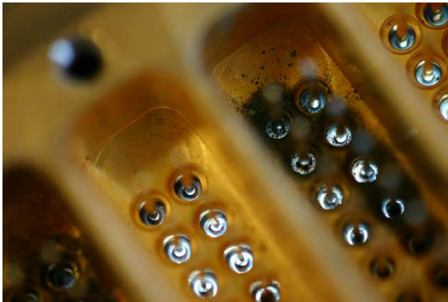
Figure 6: Corroded pin carrier from Victoria bench tests. The pincarrier is on a light table to illuminate the glass bead insulating the pin from the pincarrier body. Note the corrosion debris on some of the glass beads in the bottom picture.
