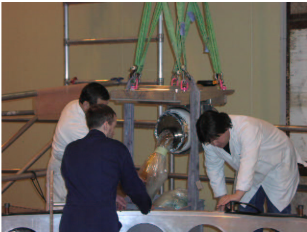
Fig. 2. Paul Poffenberger (front, Victoria) during feedthrough installation on the first ATLAS endcap cryostat.
